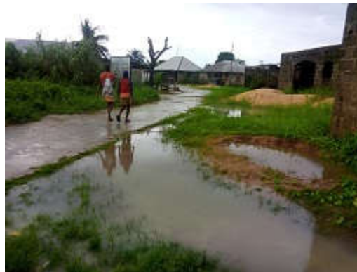
Plate 1: A dilapidated road constructed by SEEFOR just 3 years ago without drainage system, causing environmental challenge in Agbura community
