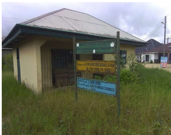
Plate 1: An Abandon cold room project in Otuokpoti Community, Ogbia built by FADAMA 111
