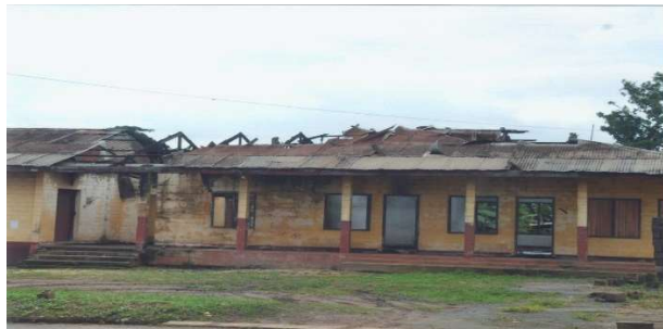
Figure 1.4 Destroyed D.O's Office Kumba Central Subdivision
